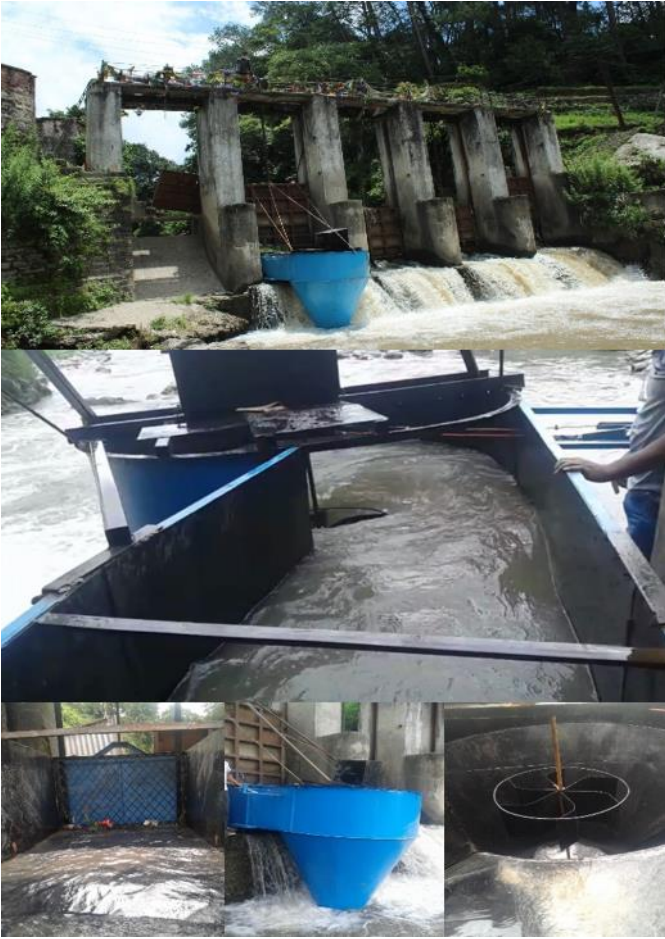
Figure 5. Pilot project using conical basin structure, with integration in irrigation canal weir, intake canal, basin structure and runner.
