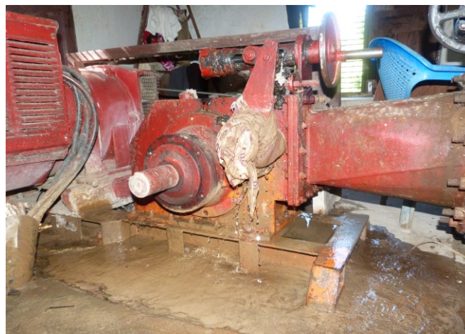
Fig. 6 Leakage from turbine casing
