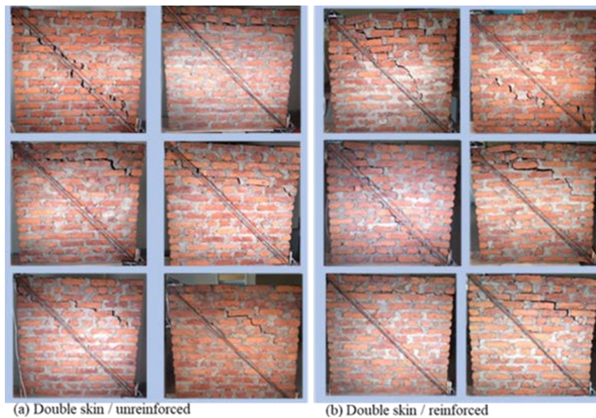
Fig. 11 – Failure mechanisms for in-plane tests on different types of panels: (a) unreinforced and (b) reinforced double-skin walls.
