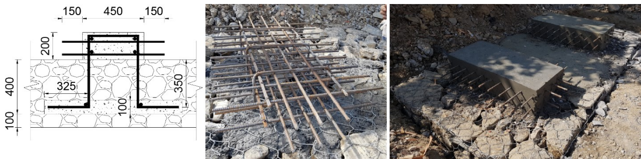
Figure 7 Cross section of the RC pedestal (left); Laid rebar before casting (mid); Casted RC Pedestals (right)
