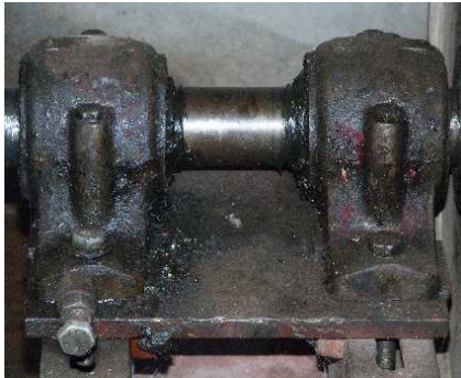
Fig. 7. Over-greasing of turbine bearings
