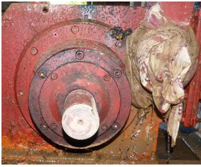
Fig. 6. Leakage from turbine casing
