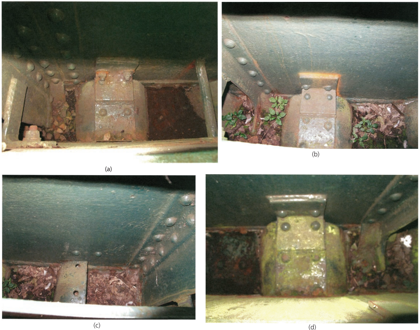
Figure 3. Angle cleat fixings showing variability due to rivet location/loss, bolt replacement, welding and fitting tolerance
